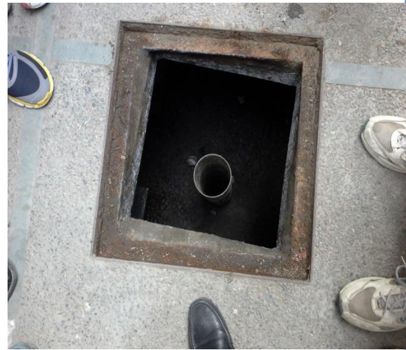
Overflow from Storm drain is directed to Sewer line – in a systematic manner
